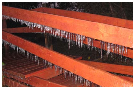
What happens when the sprinklers are left running during a frost.
